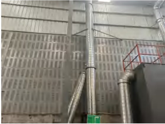
15m 排气筒 (DA007) (锻造、打磨焊接、补灰工序)
